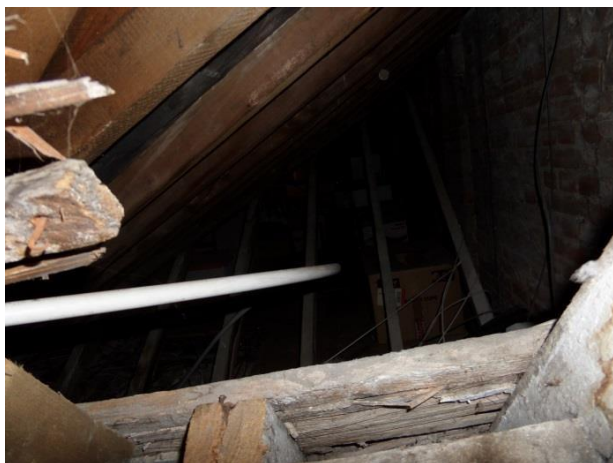
Ref: 1.4.1. Holes in loft space internal walls
