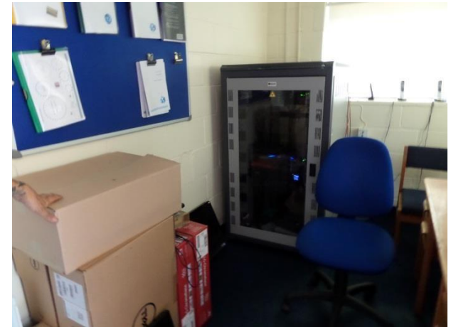
Ref: 1.2.1. Combustible material stored next to server equipment
