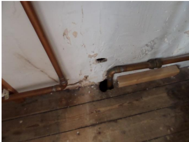
Ref: 1.4.1. Page 13. Holes in service cupboard ceiling
