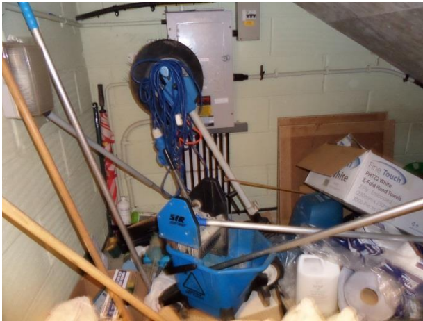
Ref: 1.2.1 Combustible material stored next to electrical equipment
