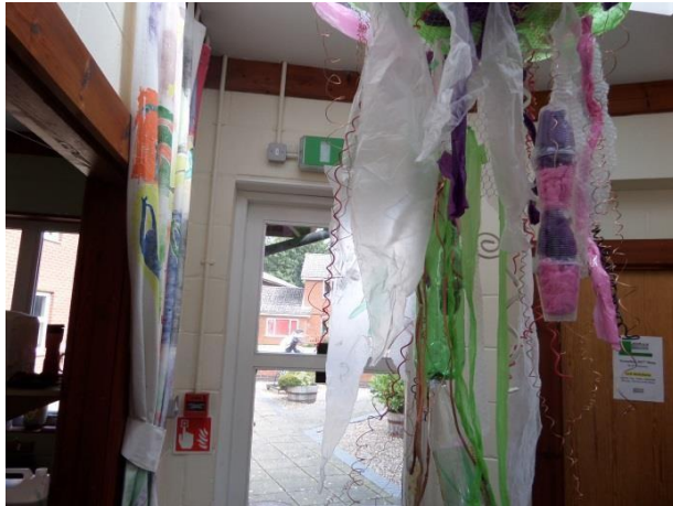
Ref: 2.2.3 Blocked Fire Exit
