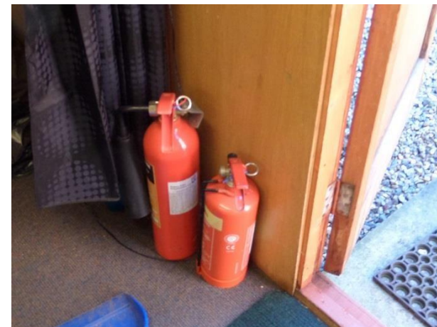
Ref: 2.3.2. Fire extinguisher floor standing and not on Fire point
