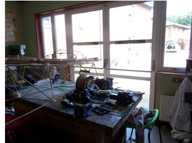
Ref: 2.2.3 Workbench blocking Fire exit
