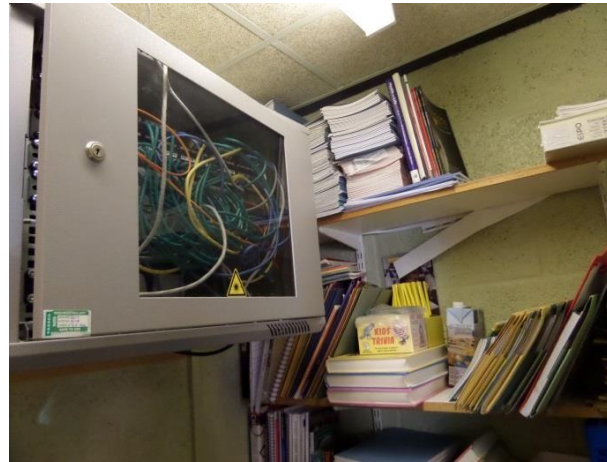
Ref: 1.2.1 Combustible material stored next to server equipment
