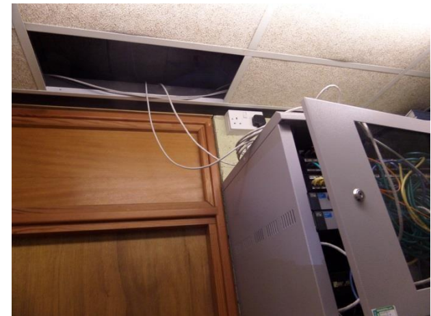
Ref: 1.4.1. Ceiling tiles missing
